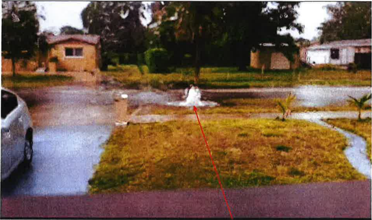
Backflow surging from pipe
