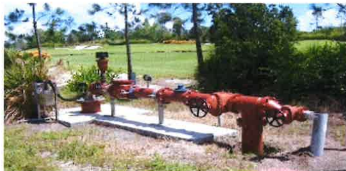
Photo 4: Surficial Aquifer Well
