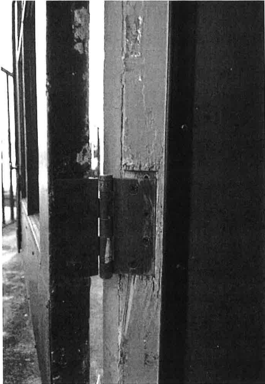
WRONG SIZE HINGE HARDWARE
