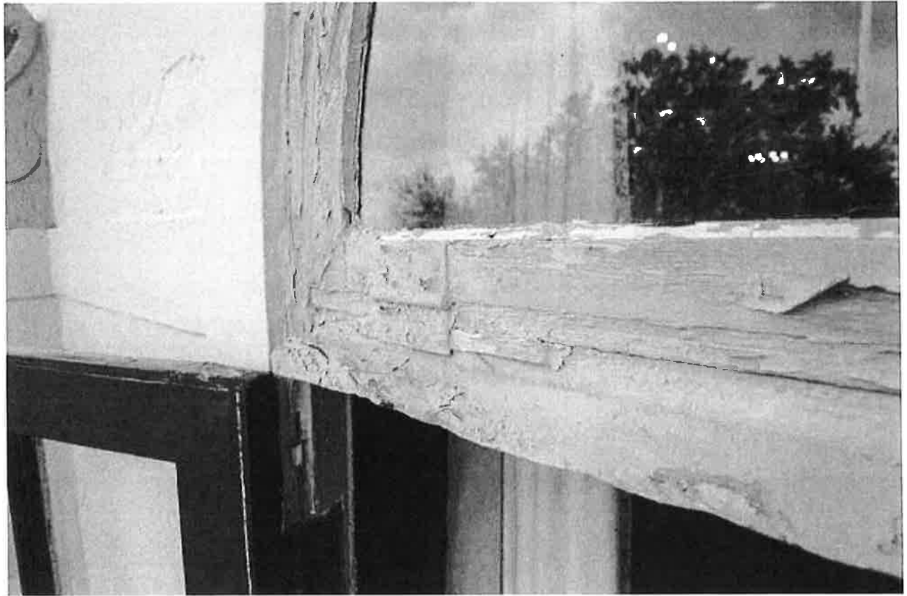
Hinges PAINTED OVER / METAL DRIP Edge
