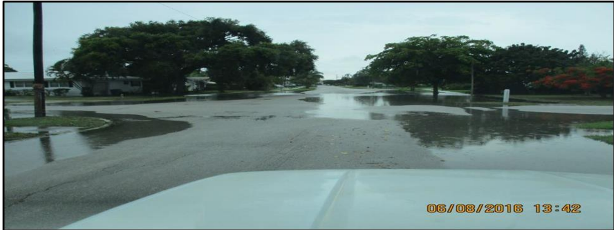
Figure 5-2 - Nuisance Flooding at 2nd Street and Ilex Drive
