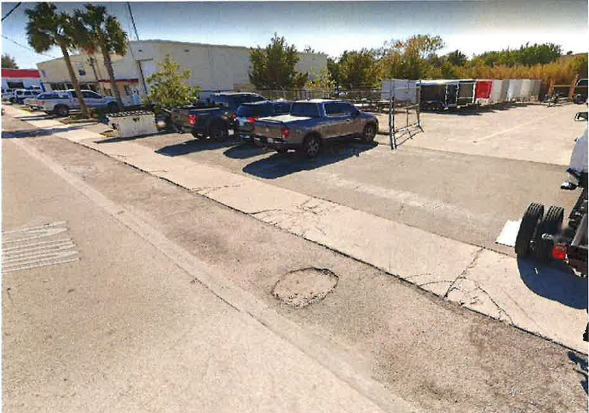
Photo: 10th Court holes in asphalt and cracked sidewalk showed unsafe conditions
