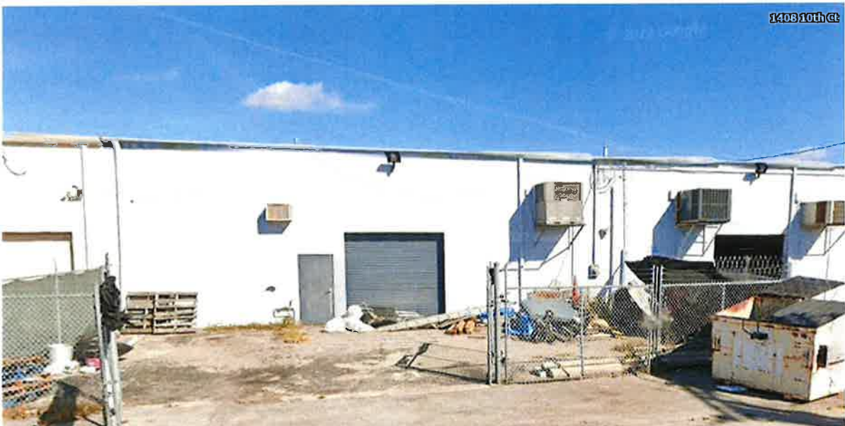
Photo: 10th Court deterioration of site improvements
