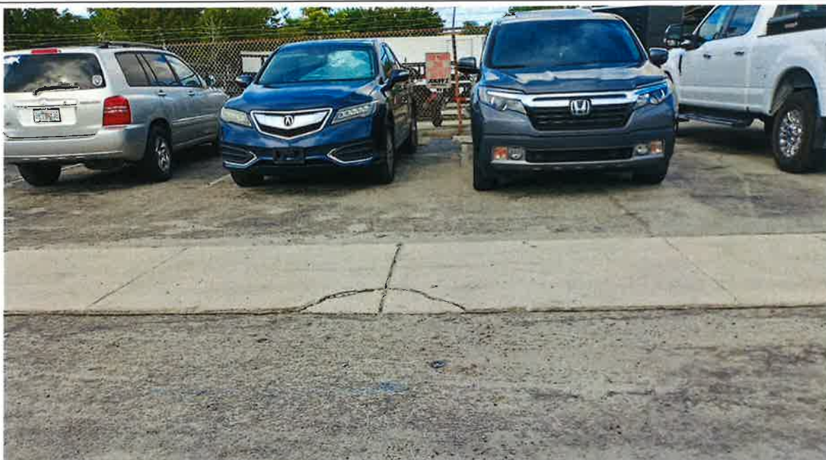
Photo: 10th Court cracked sidewalk showed unsafe conditions
