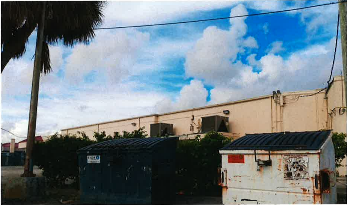
Photo: 10th Court obsolete and outdated building facade facing Prosperity Farms Road - In addition to inadequate ventilation and light.
