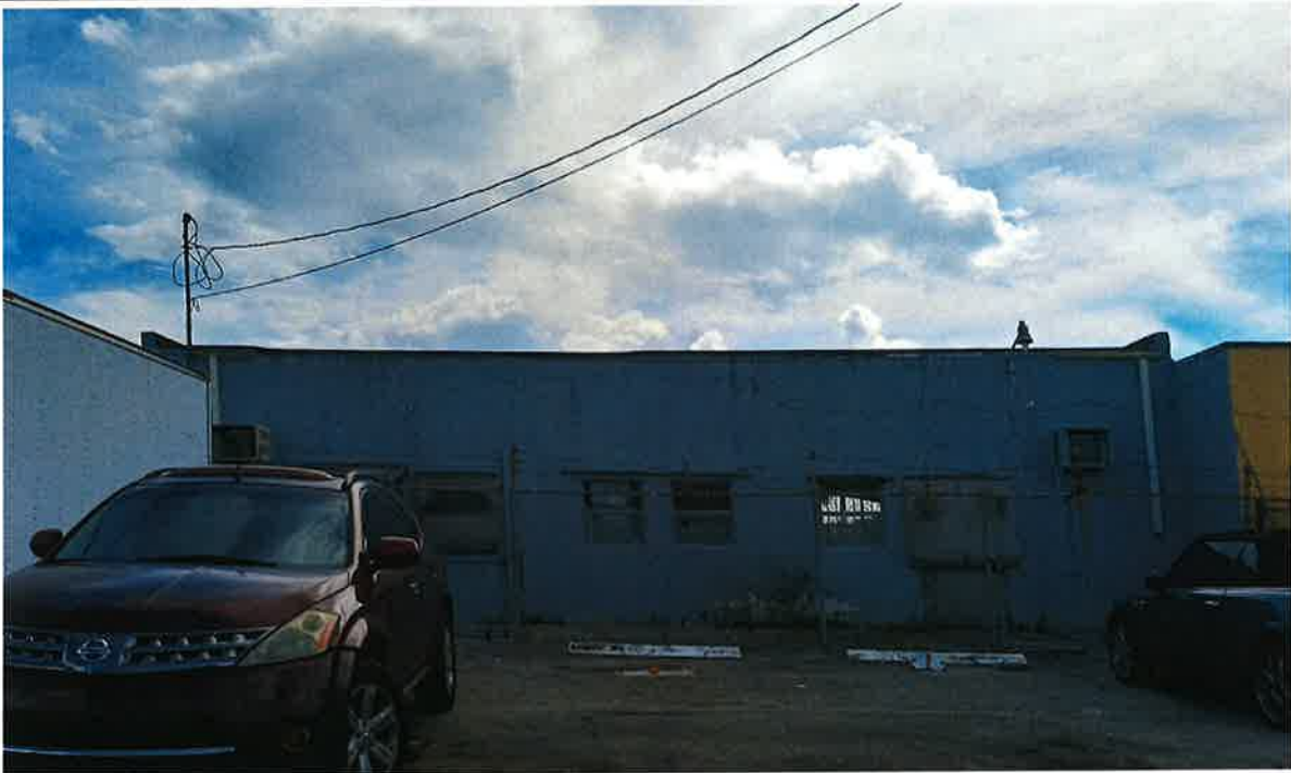
Photo: Dilapidated building structures.
