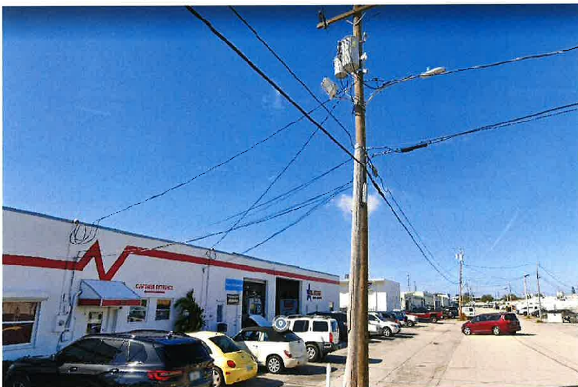
Photo: 10th Court electrical lines unsafe conditions
