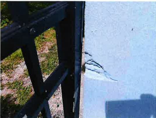
Minor Chip on Block Wall
