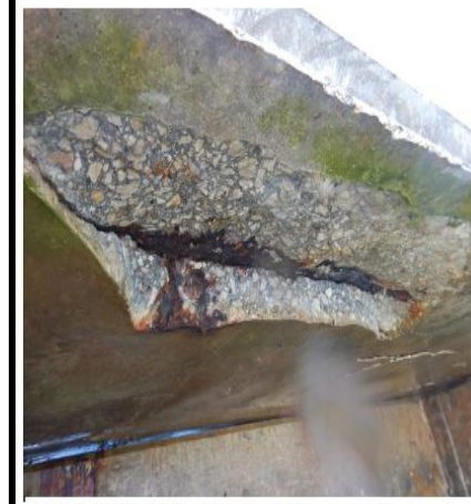
Photo A-40: Delamination at the bottom of the concrete slab between bent 14 and bent 14-a.
