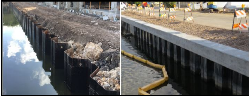
Steel Sheet Piles Bulkhead
