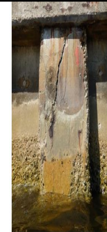
Photo E-55: Deterioration on soldier piles at the easement bulkhead.
