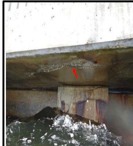
Photo A-39: Delamination on the bottom of the concrete slab at bent 13-a.
