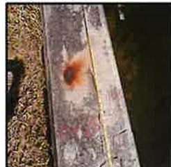
Photo E-47: Cracks and stain (blue) on concrete cap above pile 1.
