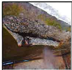
Photo A-49: Close-up of the bottom of the concrete bulkhead between pier 7 and pier 6.
