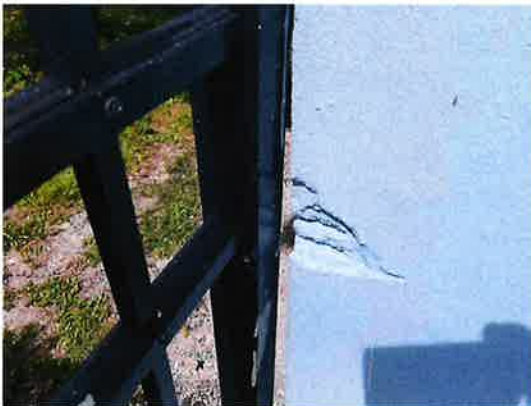
Minor Chip on Block Wall
