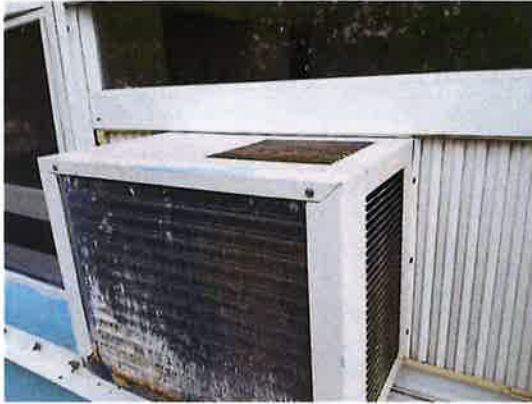
Window AC Unit
